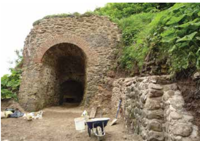
The eastern lime kiln at Hawthorn Hive, consolidated along with the retaining wall next to it which has been rebuilt using stone from the Dene.
