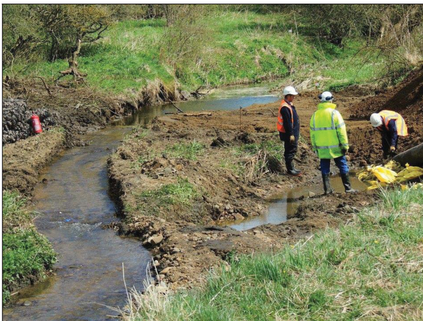
Restoring the habitat at Hetton Bogs following serious flooding in June 2013. The stream banks had been completely washed away by a water surge.
