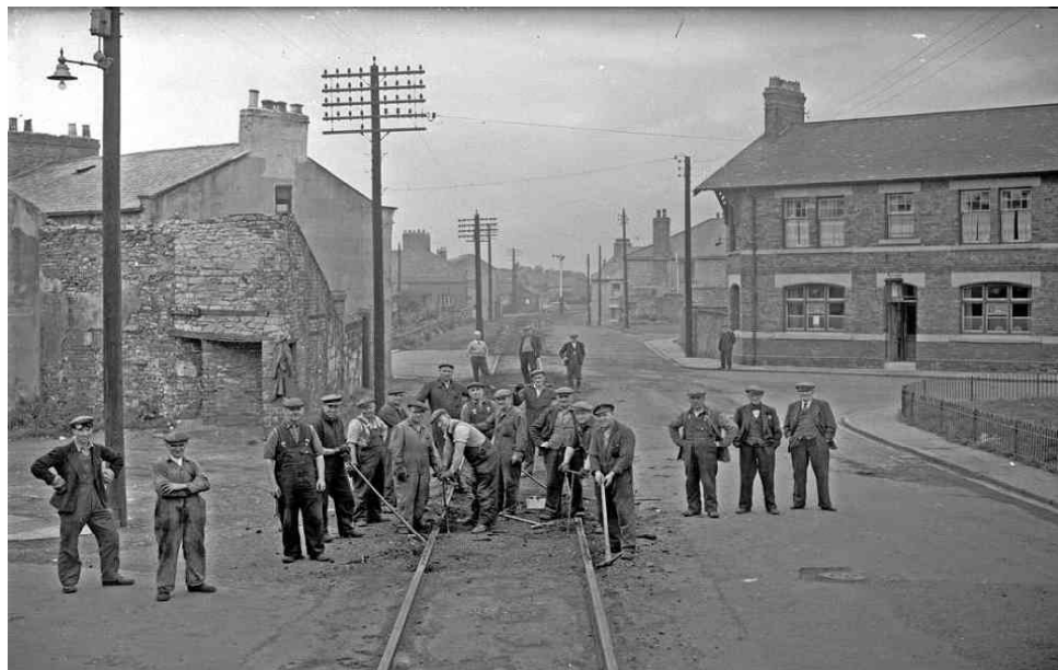
Lifting the track of the Hetton Colliery Railway in Railway Street, Hetton, in 1959
